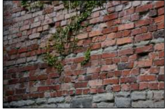
Photo 19 – Close-up of the north-west wall of the Vertical Engine House. The bottom of the wall is made of stone, with brick above. Note the single course of thin stone running across the middle of the photo.
