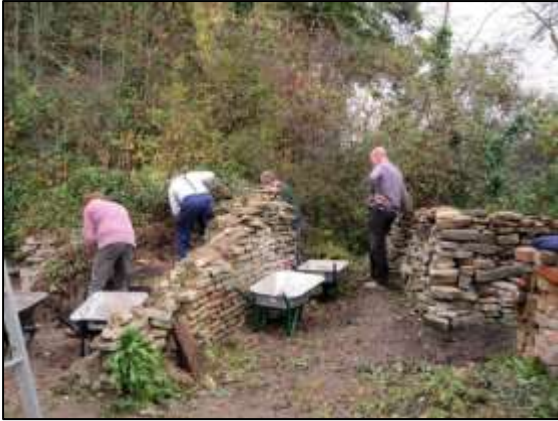
Photo 16 – Clearance work on both the inside and outside the Vertical Engine House.
