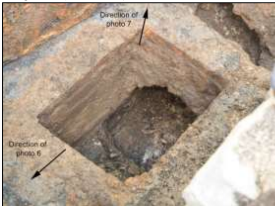
Photo 5 – Close-up of the manhole in the base of the winding drum pit, Vertical Engine House, showing the arched construction of the top of the drain.
