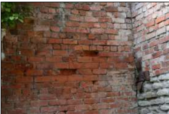
Photo 18 – Close-up of the centre of the south-west wall of the Vertical Engine House, showing the area above the winding drum pit where the bond and type of bricks change.
