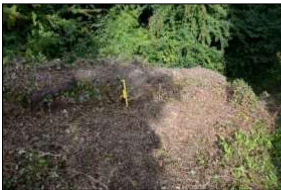
Photo 1 – The original brick raised edge of the Old Pit heapstead from the top of the heapstead. (30 cm scale)
