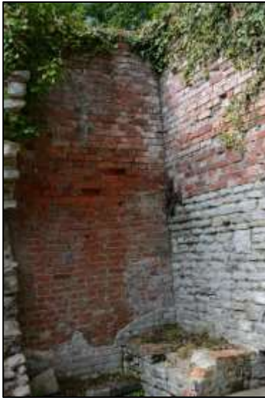
Photo 17 – Section of the south-west wall above the winding drum pit in the Vertical Engine House. The area where there is a change in the bond and of the type of bricks used is in the middle, and can be seen in close-up below.
