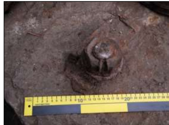
Photo 15 – This nut, one of 4 that held a cylinder down in the Vertical Engine House, has been partly cut in two with a cold chisel. A scrap of the cylinder casing, left attached to the bolt, can be seen in to the left and top of the bolt. (30 cm scale)
