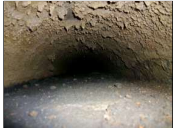
Photo 6 – View southwards along drain running under winding drum pit, Vertical Engine House. (© K Kemp)
