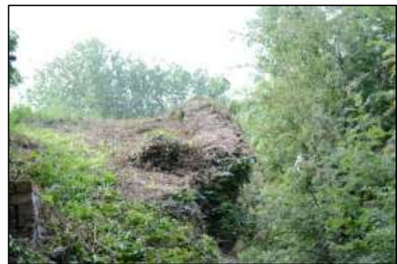
Photo 2 – The original edge of the Old Pit heapstead can be seen in the centre of the photo. The apparent overhang has been caused by the face of the heapstead wall below crumbling away.
