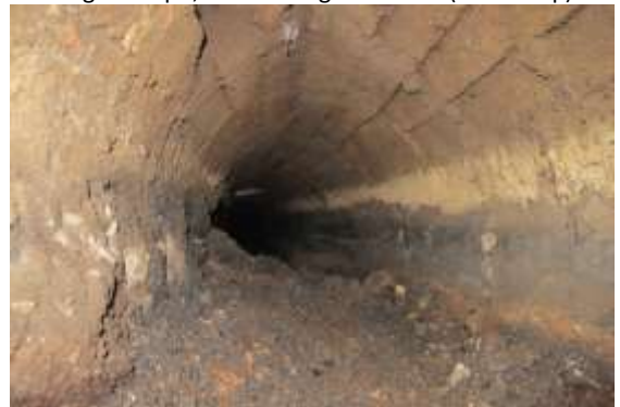
Photo 7 – View northwards along drain running from winding drum pit towards Old Boiler House. (© S Grudgings)
