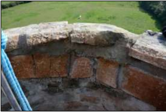
Photo 3 – Close-up of the top of the chimney during the rebuild, before the concrete ring was cast.
