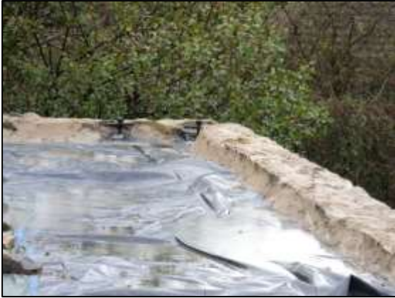
Photo 9 – Close-up of the eastern corner of the Horizontal Engine House roof, showing the rebuilt walls and an intermediate membrane in place.
