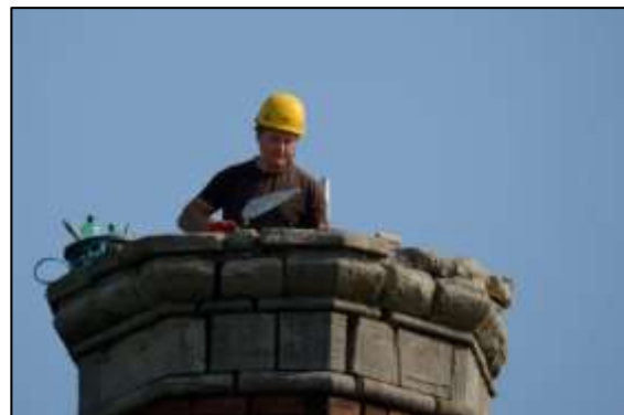
Photo 2 – One of the masons at work on the top of the chimney.
