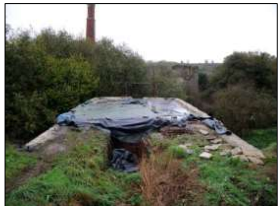
Photo 8 – Reconstruction work on the roof of the Horizontal Engine House underway at last.
