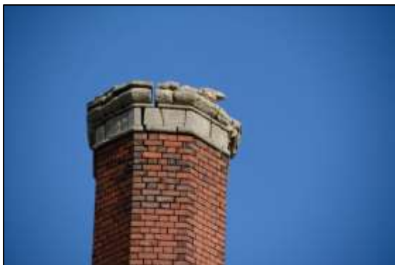
Photo 1 – View of the top of the chimney in March 2014. This was taken from about the same spot as the one of the finished top, seen on the first page.
