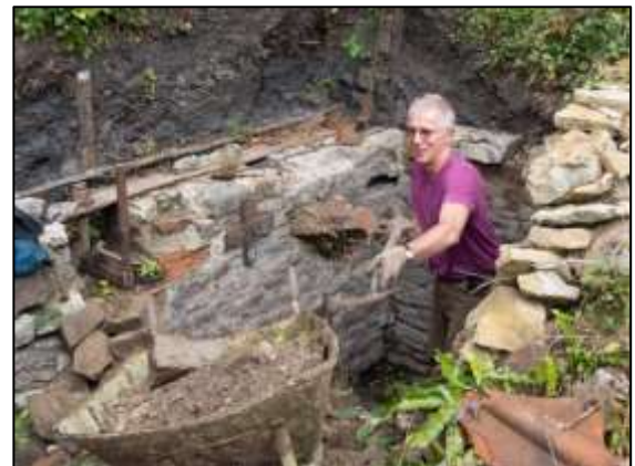
Photo 14 – The dirt is sent flying out of the winding drum pit in the Vertical Engine House.
