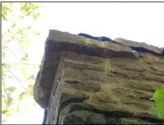
Photo 10 – Close-up of the northern corner of the Horizontal Engine House, showing the stonework placed to channel water draining from the roof away from the walls below.
