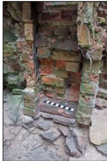
Photo 7 – Close-up of the bricked-up flue to the chimney in the Old Boiler House.
