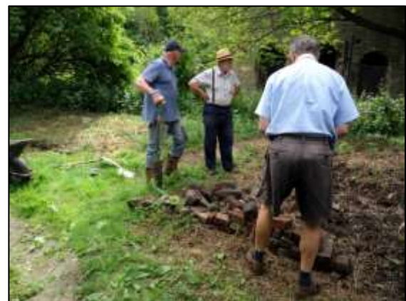
Photo 4 – Starting to clear a passage between the two enclosures for the arrival of the container.
