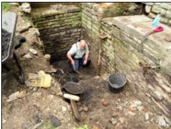
Photo 1 - Clearing the southern end of the winding drum trench in the Vertical Engine House.
