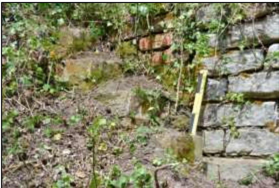
Photo 6 - Close-up of the remains of the step supports above the entrance to the Pumping Shaft passage.
