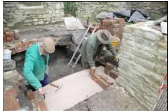
Photo 5 – Ken and Hamish start on rebuilding the arch using bricks recovered from around the site, including those found in the undercroft of the Horizontal Engine House ...
