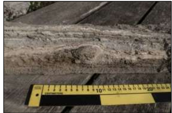
Photo 18 – This close-up of one of the pieces found in the channel in the bob wall shows how the lime scale has been built up layer by layer. (30 cm scale)
