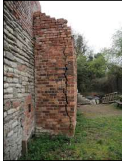
Photo 28 – Crack in the brick extension to the south-west wall of the Old Pit heapstead on 30 Mar 19. (See text on p.3)
