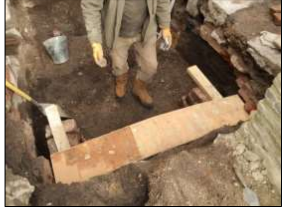
Photo 4 – The arched vault on the south-west side of the Cornish Engine House was rebuilt using this former. A second one was added later so that half of the vault could be rebuilt during a single work party.
