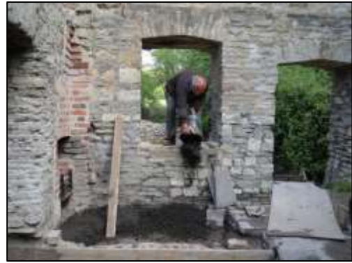
Photo 10 – Ken dumping a bucket-load of weak screed mixture onto the top of the arched roof of the north-east vault.
