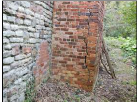
Photo 29 – For comparison this photo of the crack was taken on 16 Nov 13.
