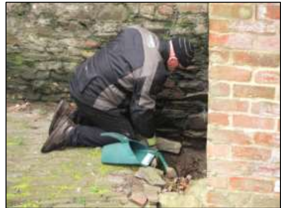
Photo 36 – Mike sweeps up the accumulated leaves in the Old Boiler House at the end of March ...
