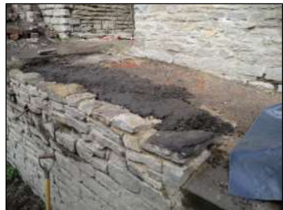
Photo 23 – The outer edge of the platform outside the south-west wall of the Cornish Engine House has been built up, and a weak screed mixture has been laid on the area behind the edge.
