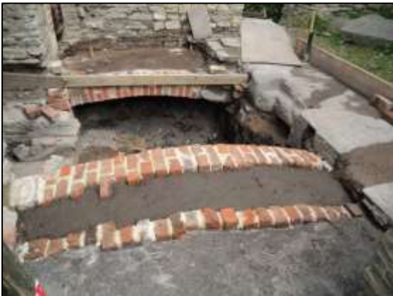
Photo 9 – The completed arch, with a layer of weak screed laid on top.
