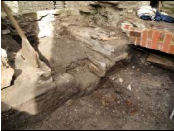
Photo 13 – An early stage in the spoil removal from the channel in the bob wall of the Cornish Engine House.
