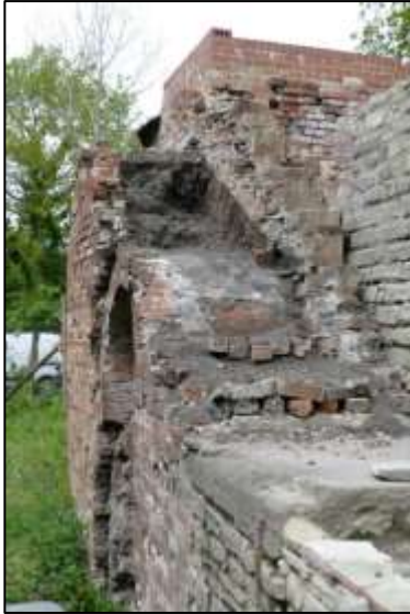
Photo 31 – Spoil has been removed from above the entrance to the Pumping Shaft passage, and part of the area behind the brick wall at the end of the Old Pit heapstead. (See text on p.3)
