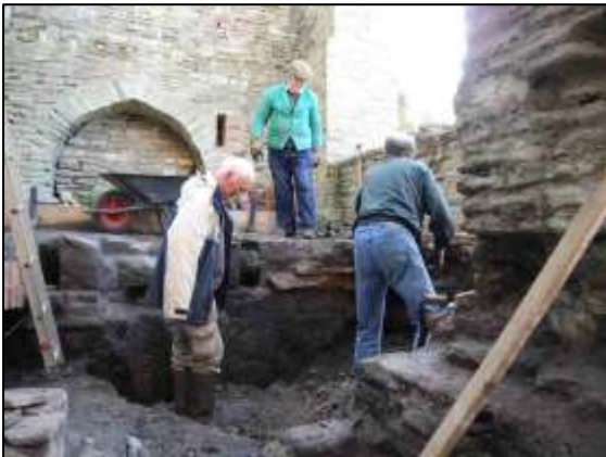
Photo 2 – Mick, Ken and Pete working on spoil removal from the inside of the Cornish Engine House.
