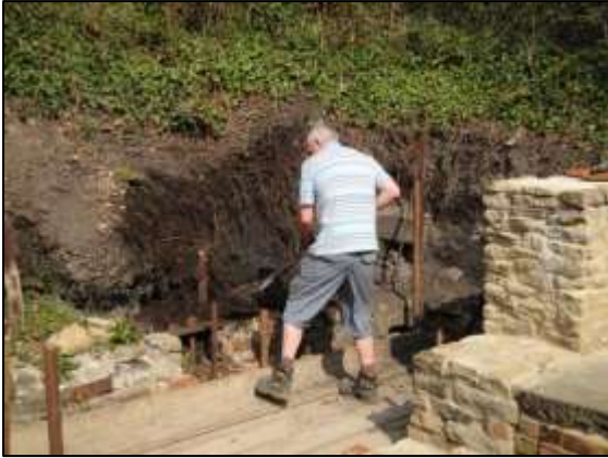
Photo 25 – Mark gets stuck into the task of clearing spoil from behind the north-west wall of the Vertical Engine House ...
