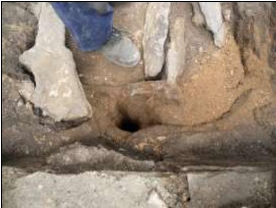
Photo 21 – Drain hole discovered at the Pumping Shaft end of the channel in the bob wall of the Cornish Engine House. (See text on p.2)
