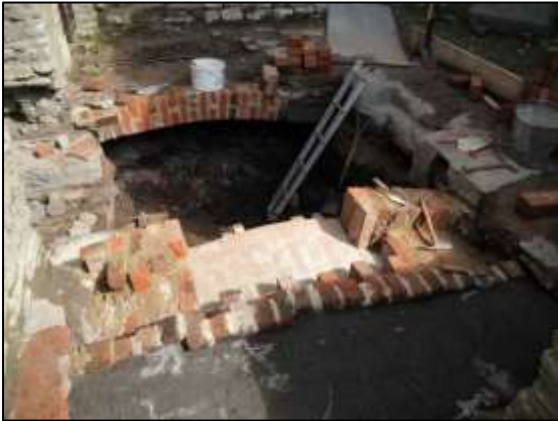
Photo 8 – A weak screed layer has been laid on the top of the first half (foreground) and work is in progress to build the second half.
