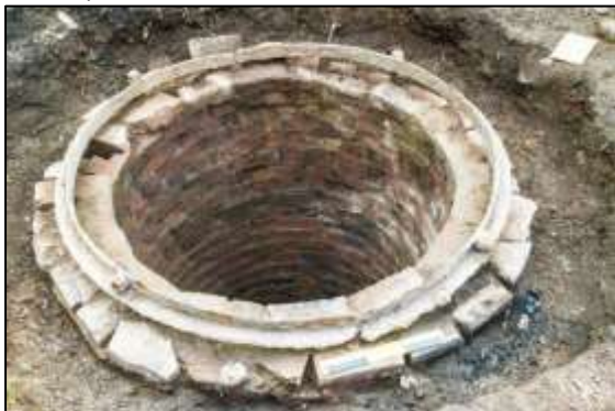
Photo 33 – The brick top of the shaft outside the entrance to the Vertical Engine House has been fully exposed, ready for repairs. (30 cm scale in foreground) (See text on p.3)
