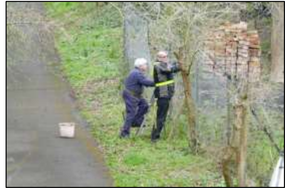
Photo 35 – Jeff and Mike repairing damage to the fence near the Old Boiler House.
