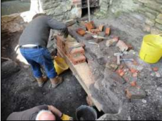
Photo 1 – Hamish building a new edge to the north-east vault of the Cornish Engine House. A view of the finished edge can be seen on p.1 .
