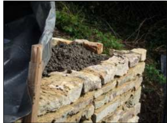
Photo 22 – The end of the wall of the platform outside the south-west wall of the Cornish Engine House has been built up, and the resulting void is being filled with a weak screed mixture.
