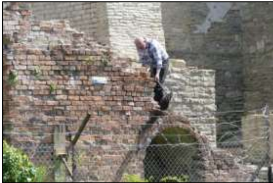
Photo 32 – Mike removes spoil from behind the wall above the Pumping Shaft passage, aiming for a wheel barrow parked out of camera shot.
