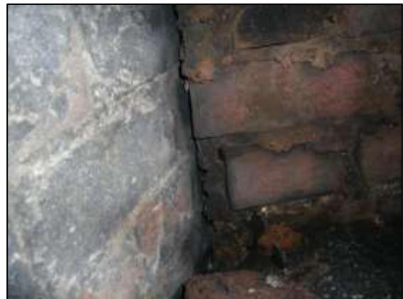
Photo 22 – View inside a cavity at the base of the north-west wall of the chimney.
