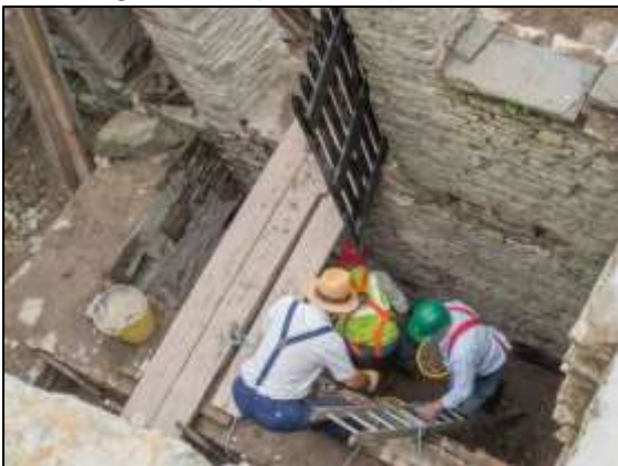
Photo 13 – Excavating spoil from the pit in the engine bay, Vertical Engine House.
