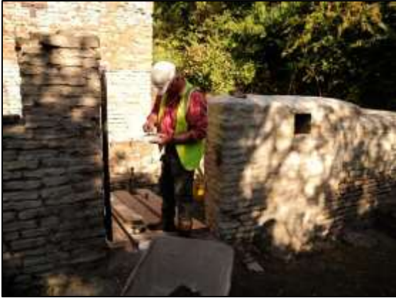
Photo 23 – Repairs being made to the gate into the Vertical Engine House after a visit by vandals.
