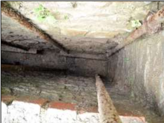
Photo 18 – North-east end of flywheel slot, Vertical Engine House, after the spoil had been cleared.
