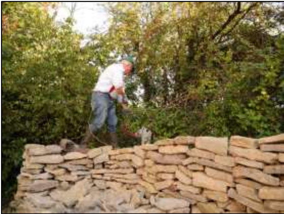
Photo 24 – Repairs being made to the fence by the Vertical Engine House after it was cut by vandals.
