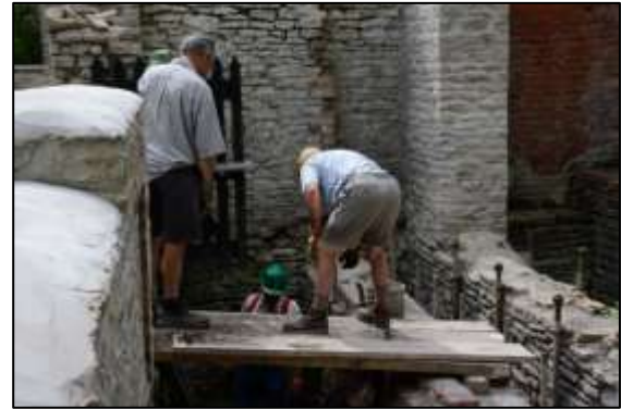
Photo 23 – Clearing spoil from the south-west end of the engine bay, Vertical Engine House ...
