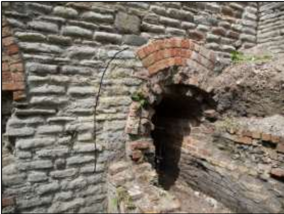
Photo 12 – The black line has been drawn around the outline of a possible structure around the entrance to the East Flue (see text).
