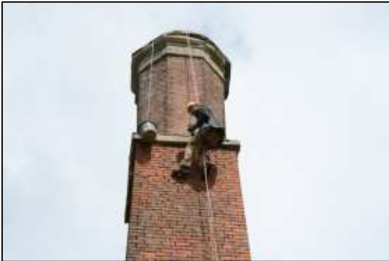
Photo 6 – Pointing in progress around new stonework at the shoulder of the chimney.
