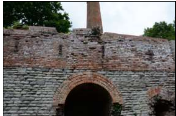
Photo 11 – South-eastern wall of the Old Pit heapstead, showing the position of the two spreader plates above the alcove.
