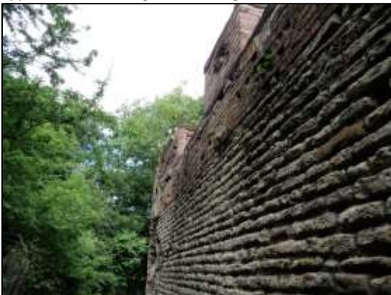
Photo 2 – the same stretch of wall after rebuilding was completed, with the pillar between the tippler slots at the top of the photo.
