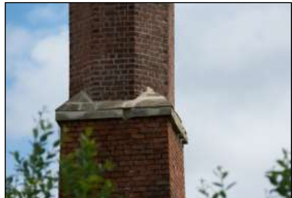
Photo 3 – The shaped stones on the shoulder of the chimney have been replaced in their original places.
