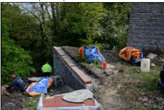
Photo 13 – Capping of the wall above the Old Pit heapstead ramp almost complete on 14 May 16 ...
