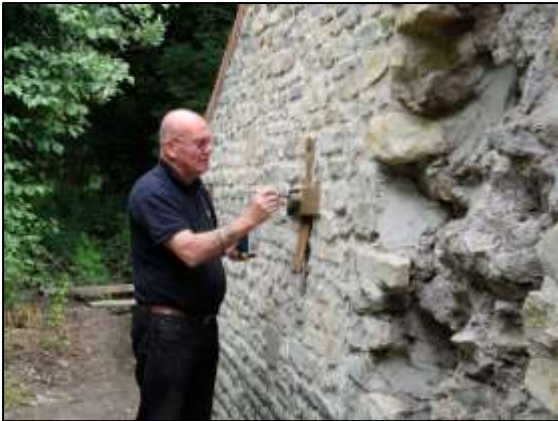
Photo 25 – Metal fittings on the Old Pit heapstead wall are given a protective coat of paint ...
