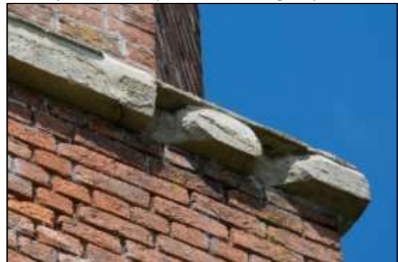
Photo 4 – Close-up of the south-east shoulder, showing where some stones were missing ...
