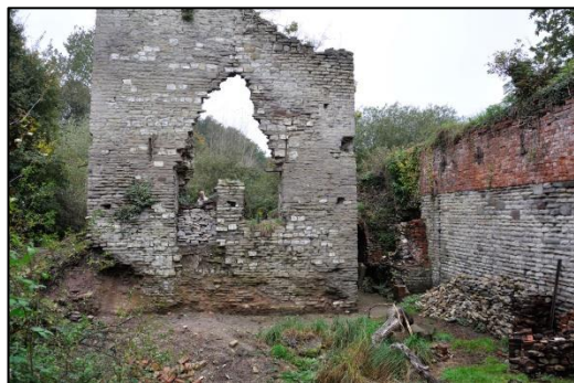
North-east wall of the Cornish Engine House at Brandy Bottom in 2011 before rebuilding by contract masons.
