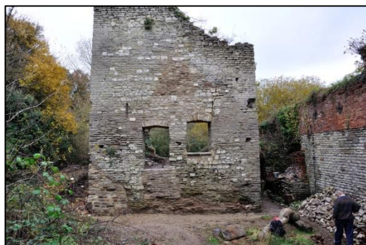
North-east wall of the Cornish Engine House at Brandy Bottom in 2011 after the rebuilding.
