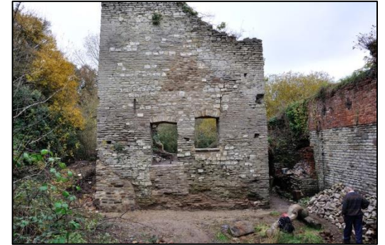
North-east wall of the Cornish Engine House at Brandy Bottom in 2011 after the rebuilding.
